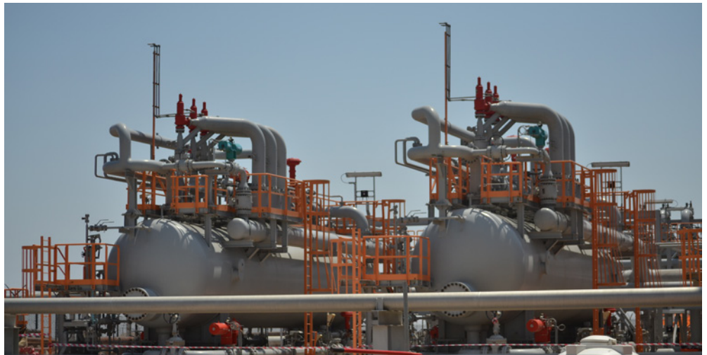
The Shamiya degassing station at the Rumaila oil field on April 29, 2019.
